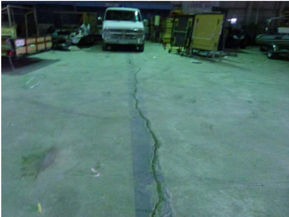
Crack noted in floor of arena.
