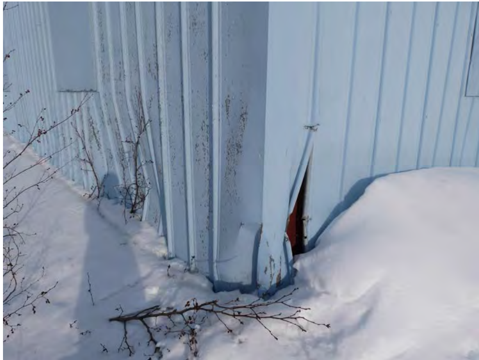
Damage to building exterior.
